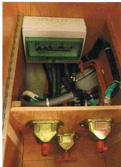
The electrical system is neat and accessible. This battery-switch arrangement was designed specifically for the test boat and will now become standard
